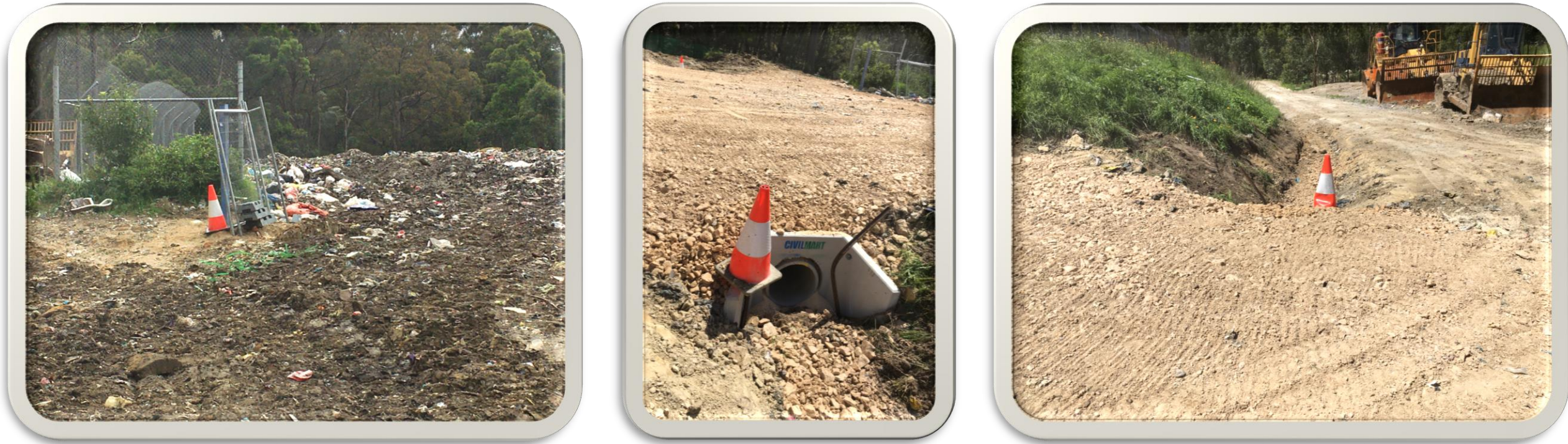
Figure 4, 5 & 6 Before and After images of drainage restoration work at Boonoo Boonoo January 2021
