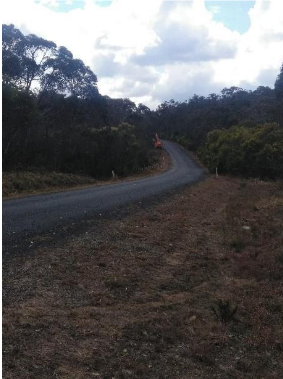
Mulching the road verge between Mursons Ck and Liston on the Mt Lindesay Rd.
