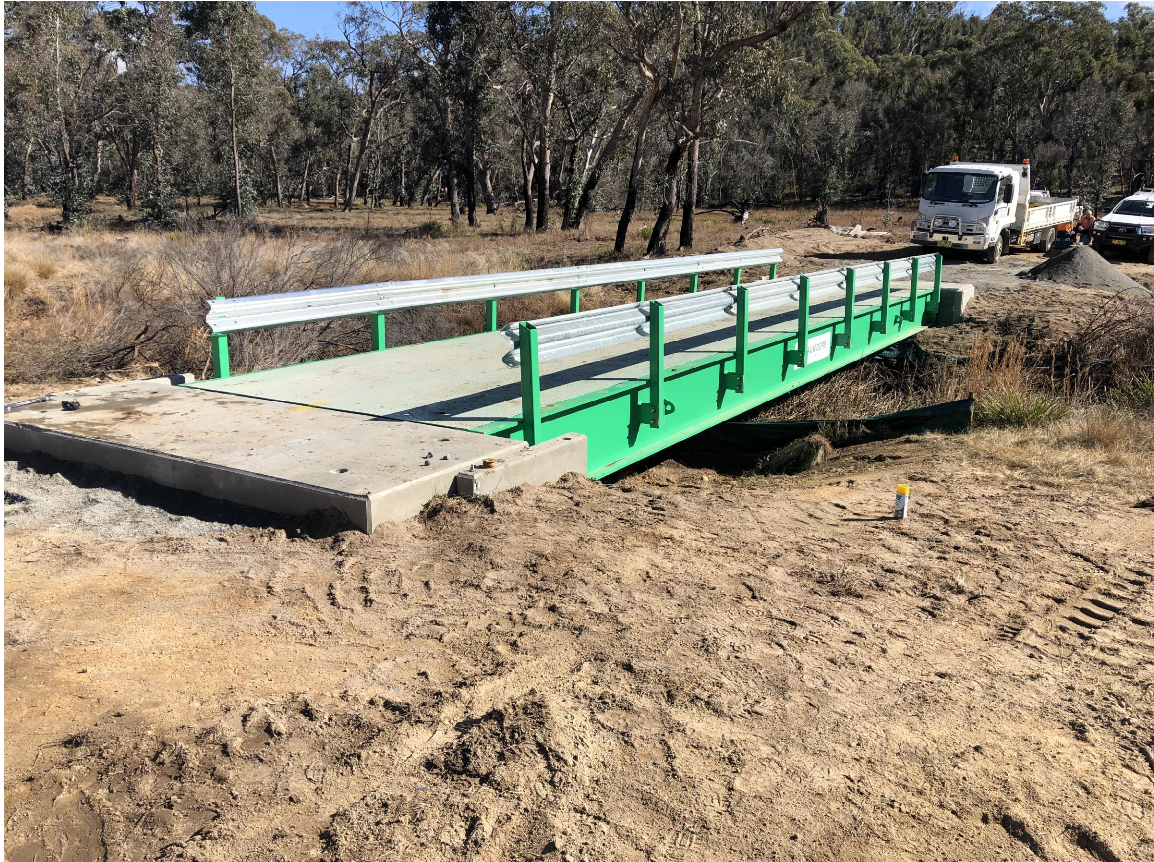
Boonoo Boonoo Sidetrack - Bridge installation – all precast abutments, wing walls and relieving slab.
