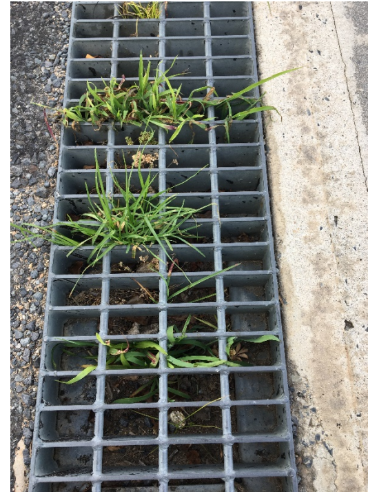
Weeds in drains
