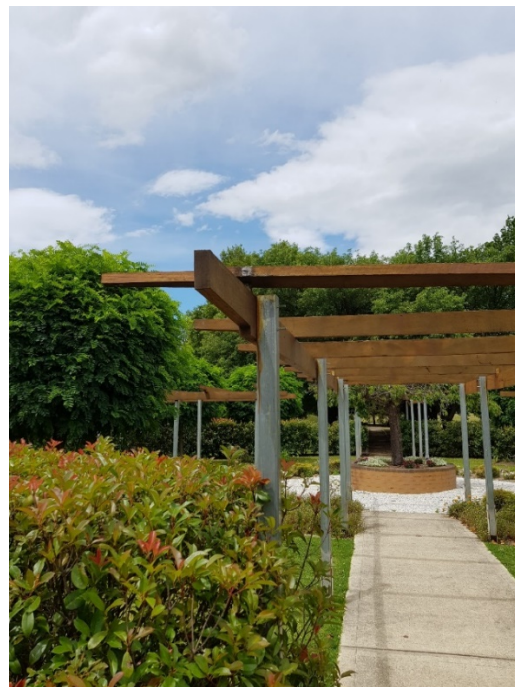
Millbrook Parks structure broken still not repaired
