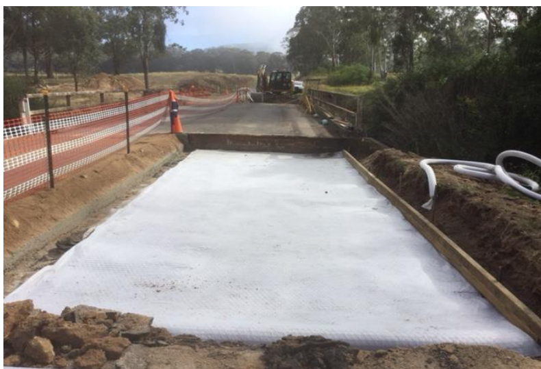
Subgrade treatment at the approach to a substantial drainage asset just north of Legume
