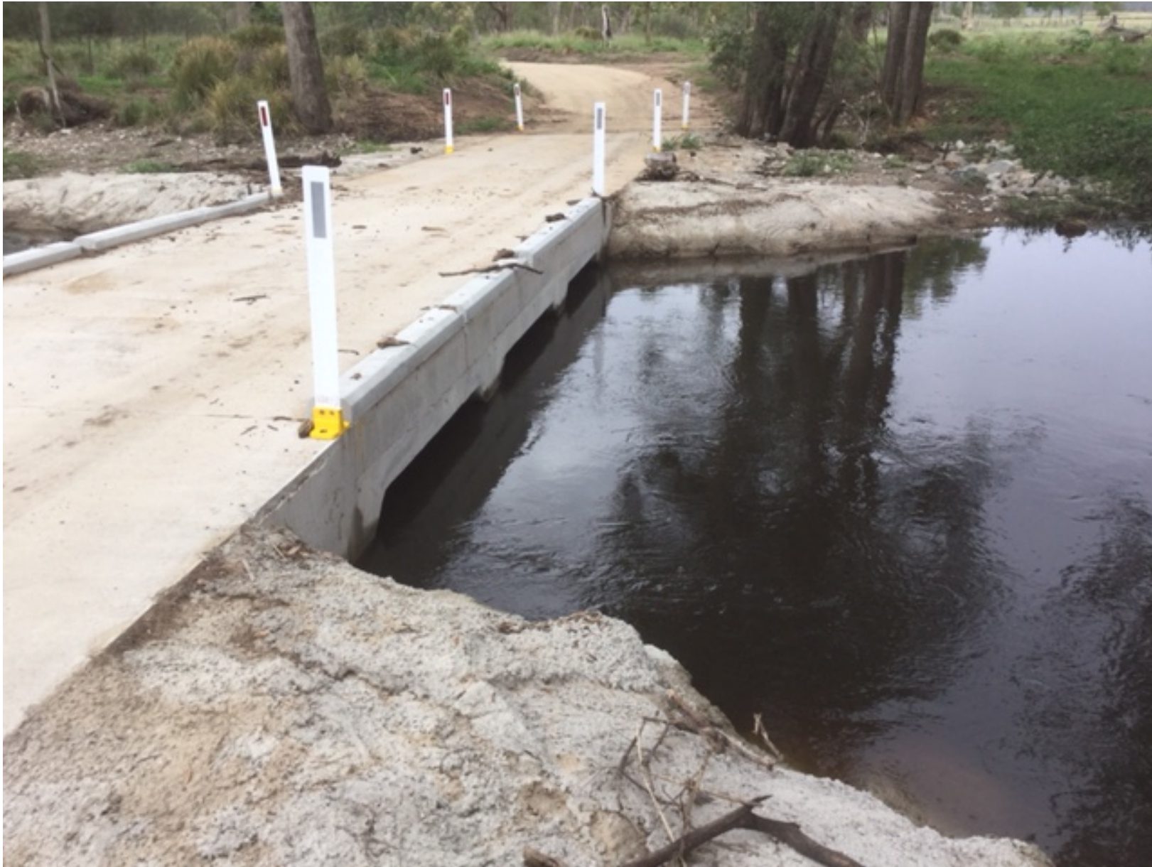
Completed culvert/ causeway on Sawyers Gully Road – after a fresh in the river!
