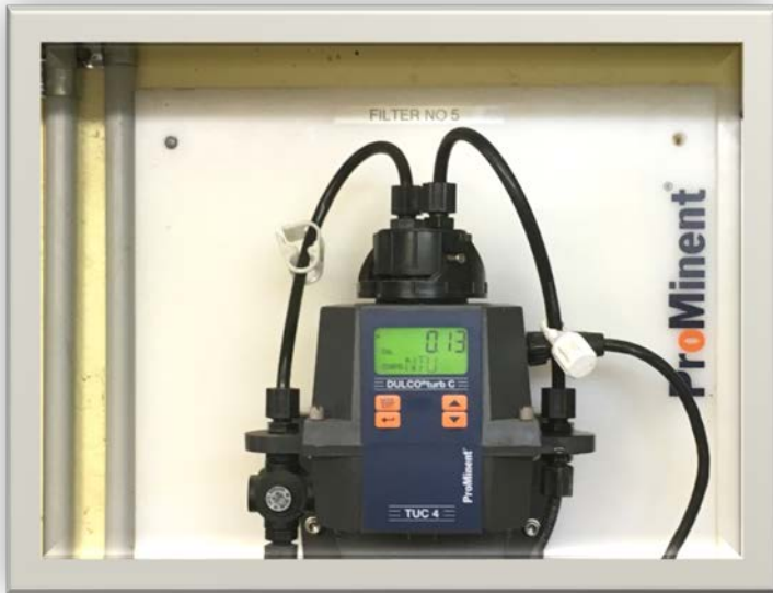
Figure 18, 19 & 20 New on-line turbidity meters installed December 2019.
